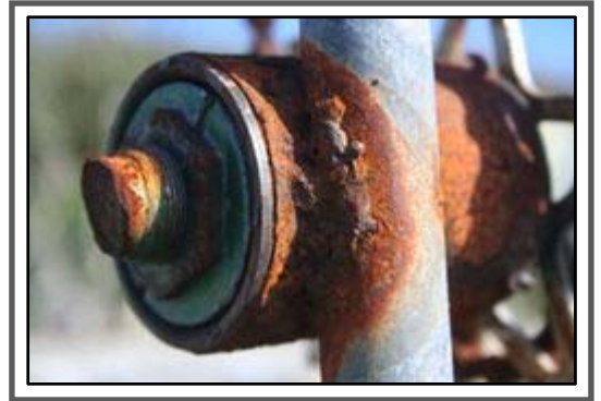
Rusting of Iron
